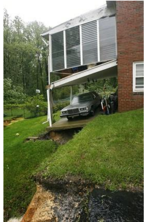
Figure 74. May 2008 sinkhole event
