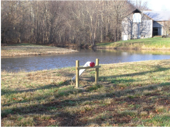
Dry hydrant in farm pond
