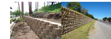
Retaining Wall-Character & Detail All Collection of All Palisades Style All Collection of All Palisades Style
