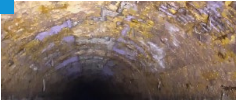
102" Anacostia Sewer Main Corrosion
