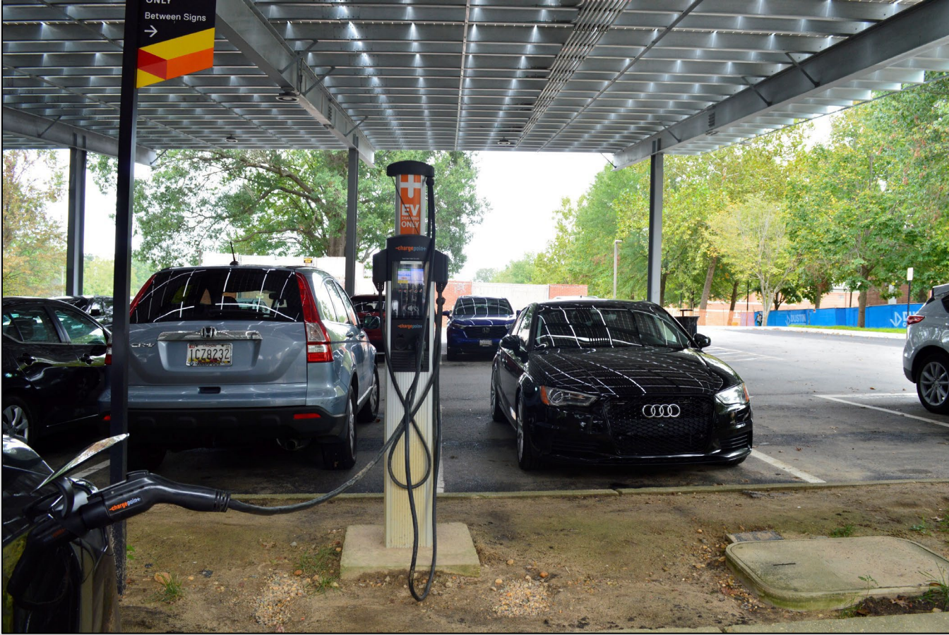
View of EV Charging Station
