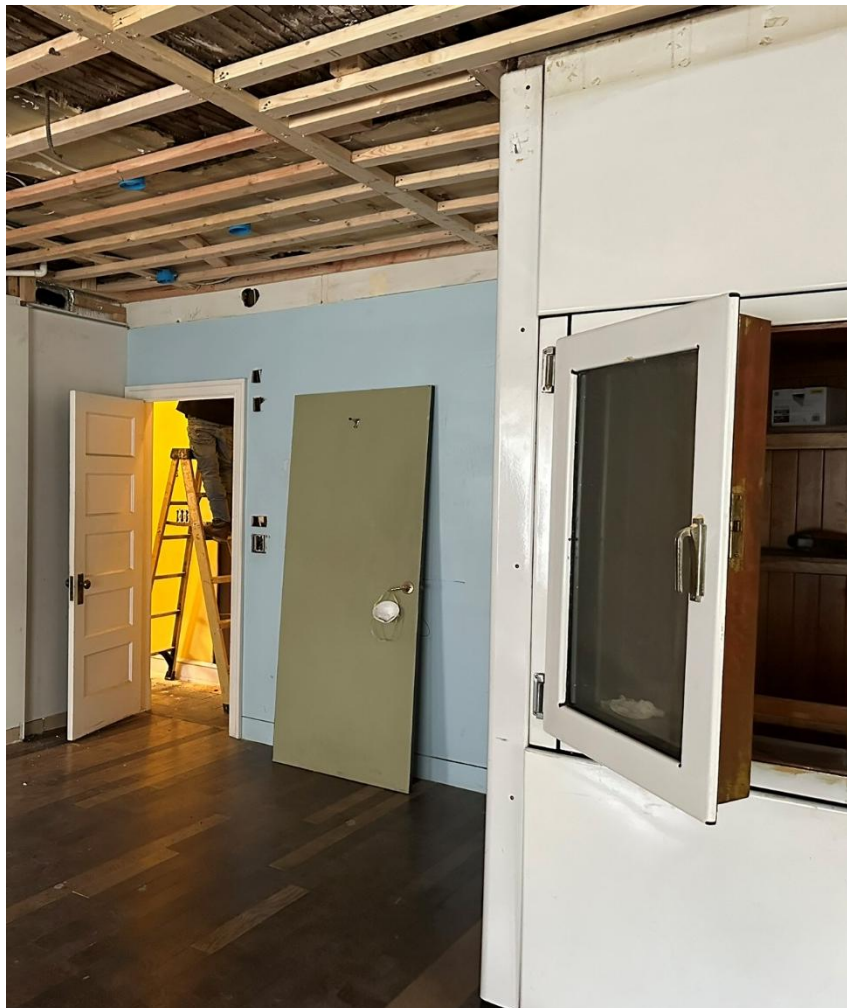
Weinstein House/Harry's Market, Interior of Store, Walk-In Cooler and Entrance to Dwelling, November 25, 2025
