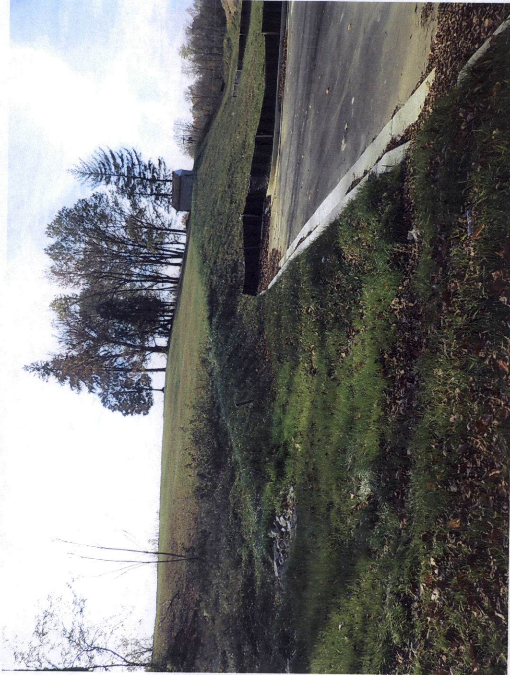
Image of the rear of the site from partially constructed Victorianna Drive
