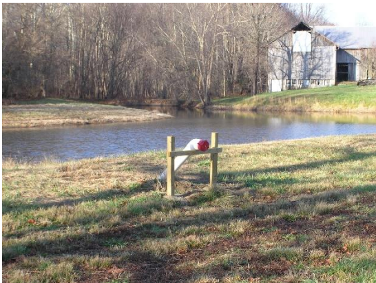
Dry hydrant in farm pond
