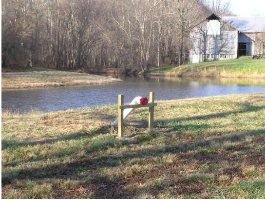
Dry hydrant in farm pond
