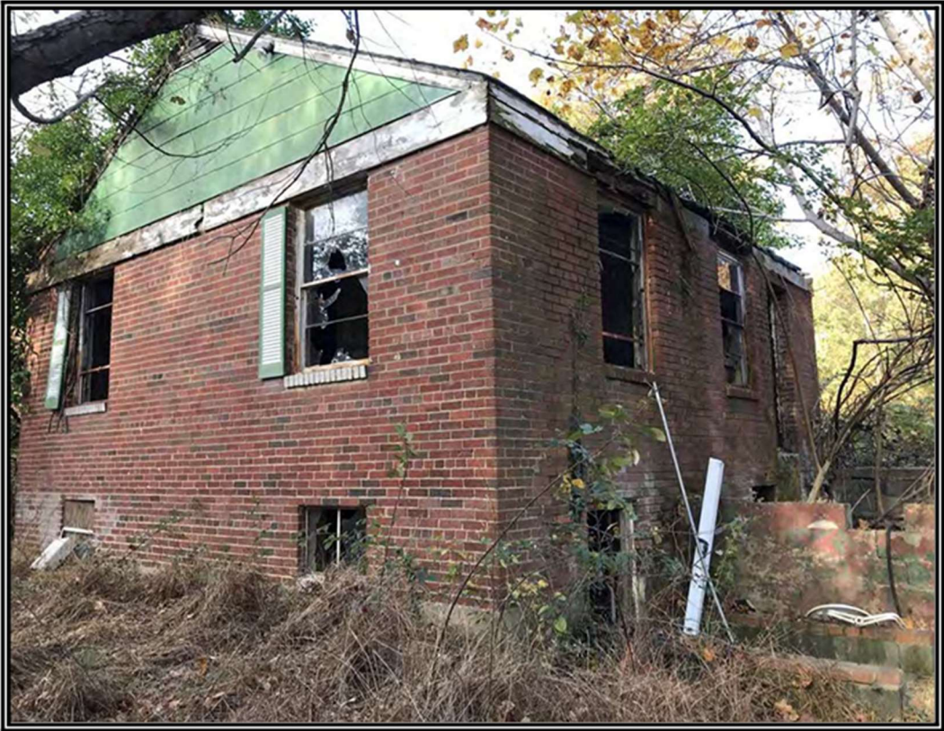
Figure 4-9. Photograph Depicting the Side and Rear of the 1940's Butler Family House (Structure 1) [facing southwest]
