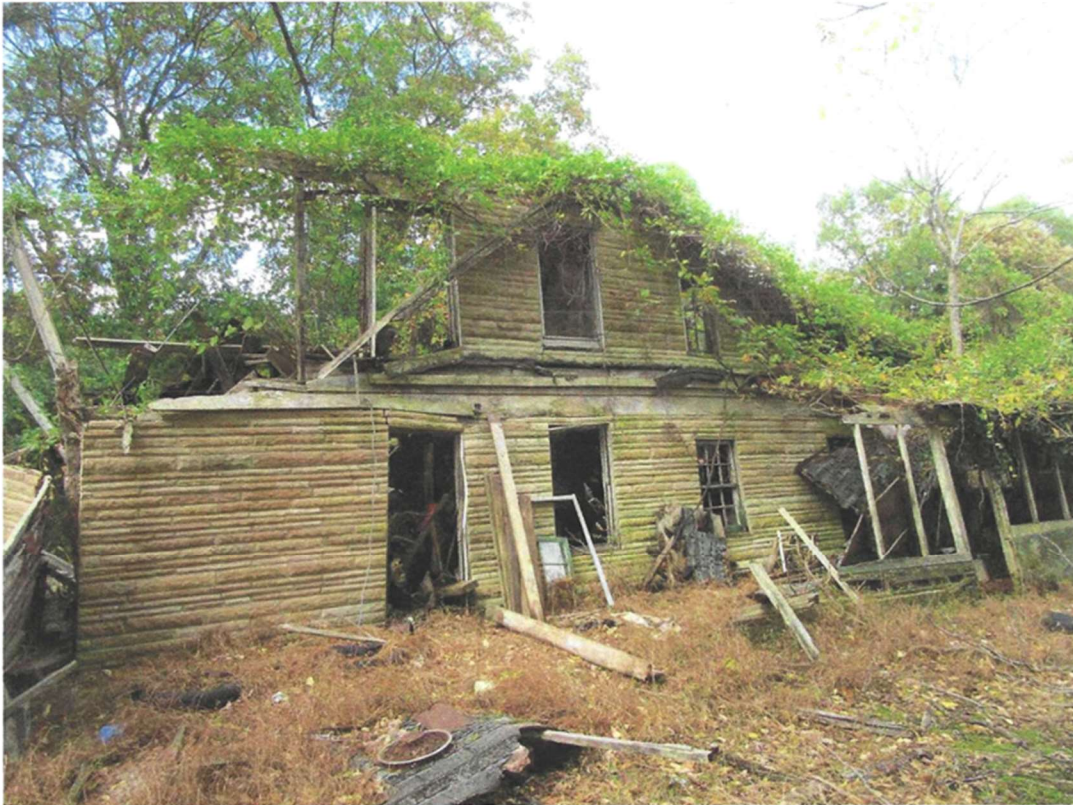
Photograph of the ruinous condition of the 1851 Butler's house
