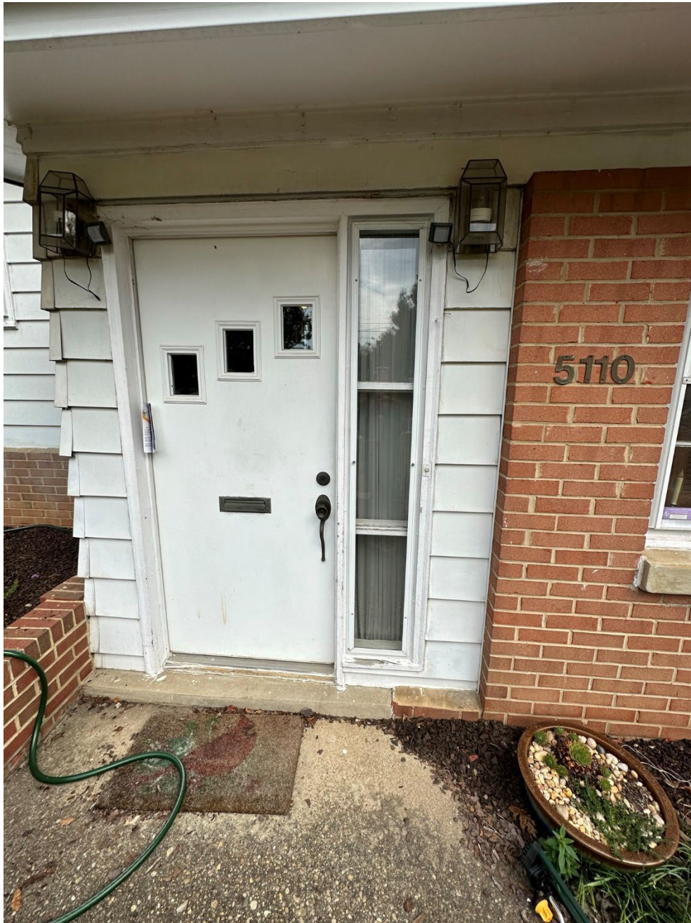
Figure 2: The entryway composition on the south elevation of the home at 8002 54 th Avenue.
