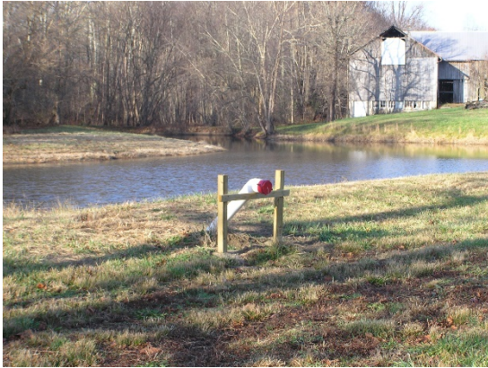
Dry hydrant in farm pond
