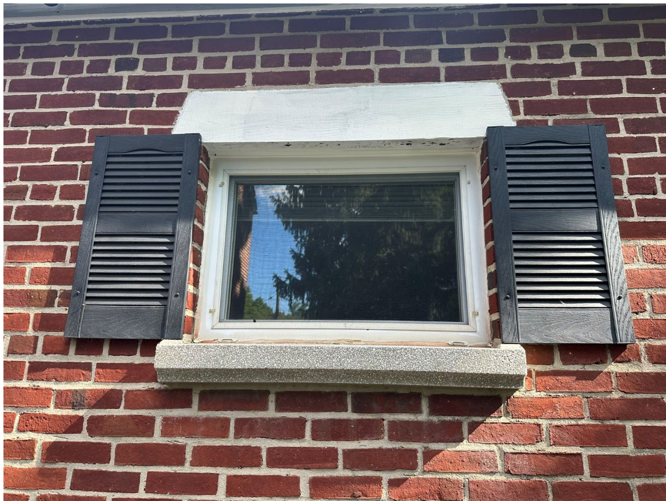
Detail, south elevation of garage showing a typical window with wood lintel and concrete aggregate sill, June 24, 2024.
