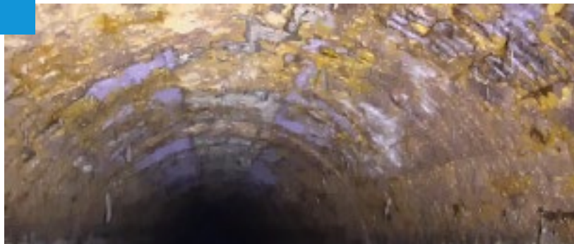
102" Anacostia Sewer Main Corrosion
