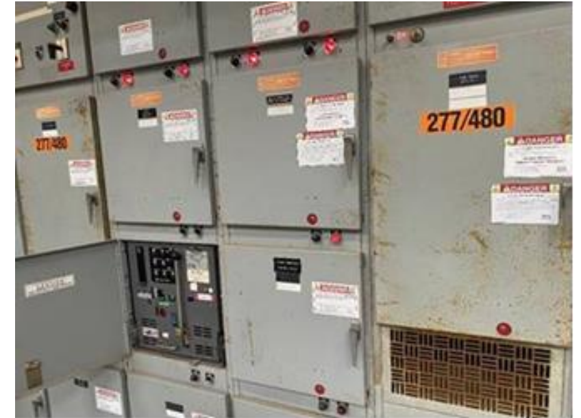
Potomac WFP Pump Station 2
